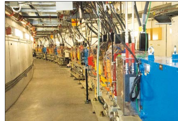
View of a double-bend achromate cell in the accelerator tunnel.
